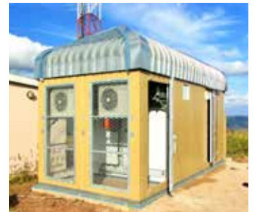
Picture: Equipment Shelter
