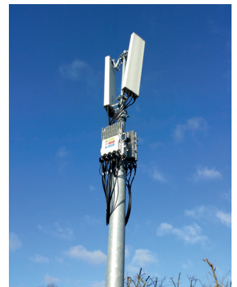
5G base station
